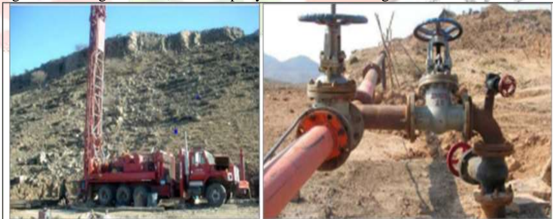
Fig. 4-3 Left: Drilling T685WS gadding machine and Right: Boreholes connected with injection pipes on the surface of the mine [13]
